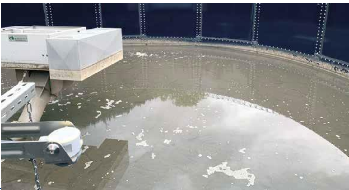
NeoWaterFX300 in use in an SBR reactor (Switzerland)
